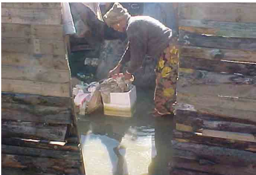
Water seeps through the floor of the houses
